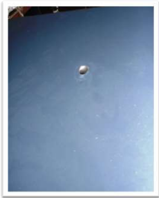
Marquee with hole for antenna
